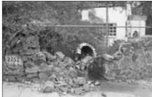
The severe damage to the grotto caused by a moving truck.
